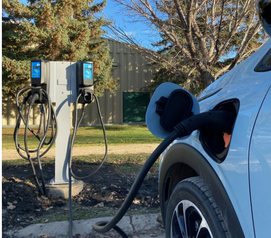
Electric Vehicle Charging Station
